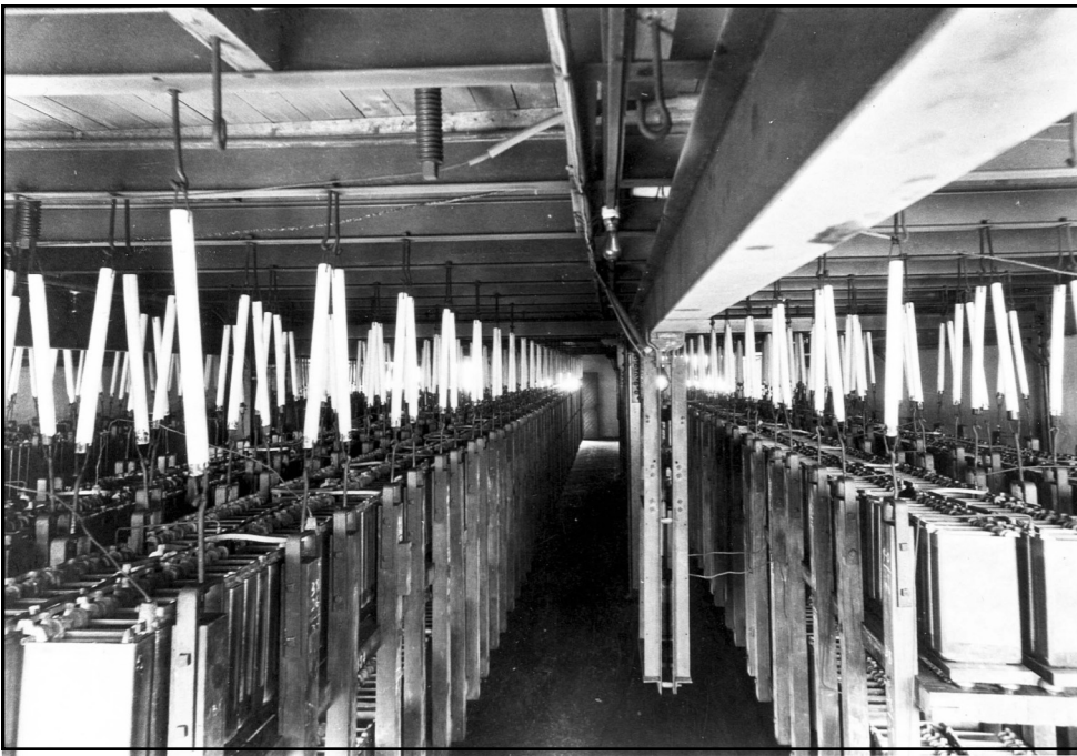
The standby battery at Marconi Towers contained 6000 two volt cells connected in series to produce 12,000 volts. It could power the transmitter for several hours if the DC generators broke down.
